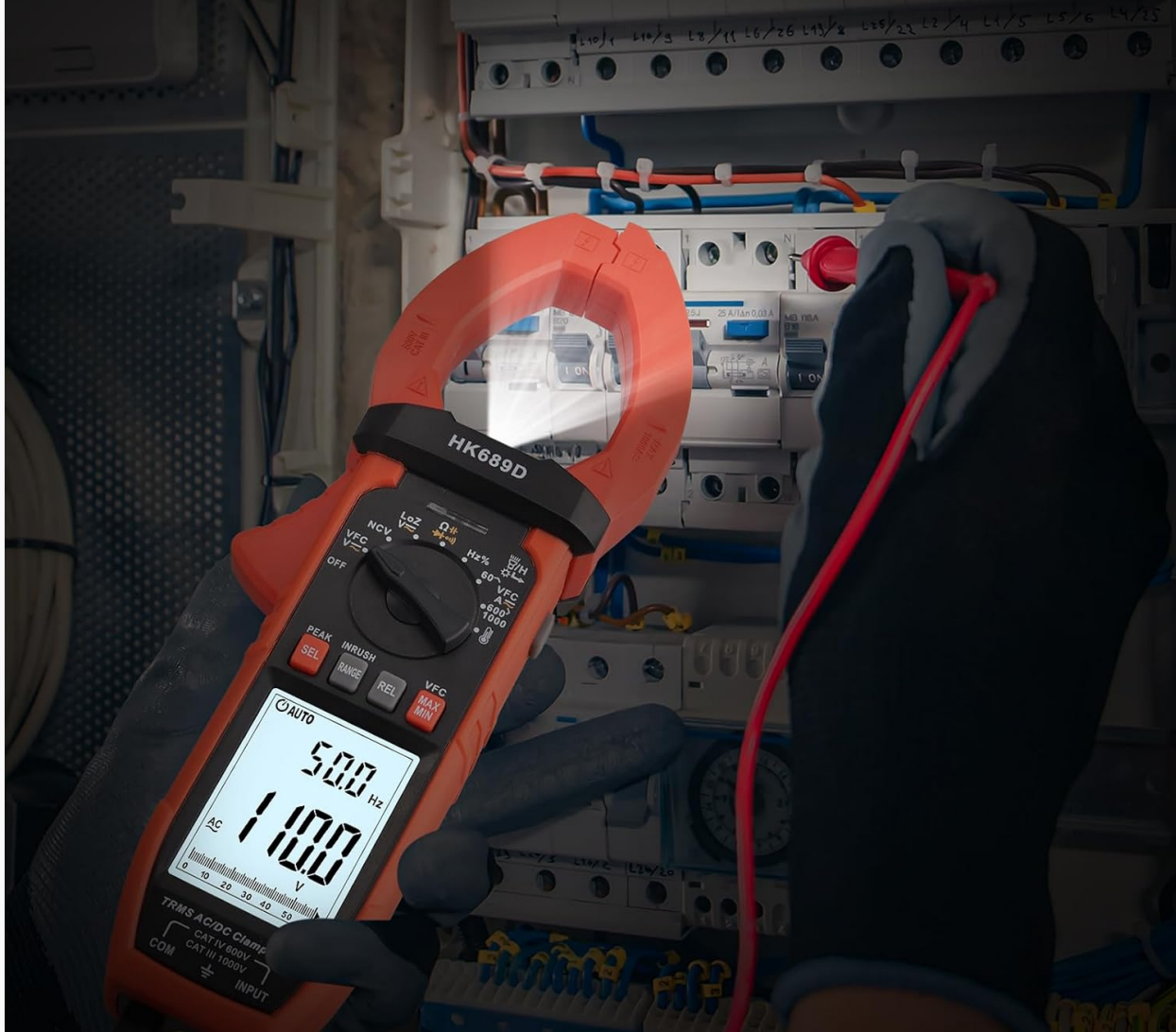
Figure 4.5: The PROSTER Clamp Meter in a dimly lit electrical panel, demonstrating its backlit display and integrated flashlight for improved visibility during measurements.
