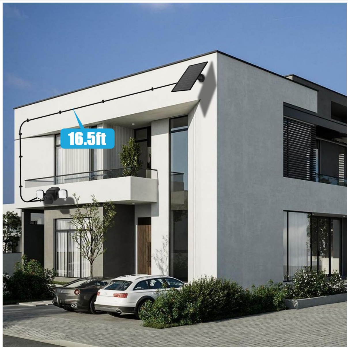
Figure 4: The UYODM 10W Solar Panel installed on an exterior wall, providing power to the Blink Floodlight Camera.
