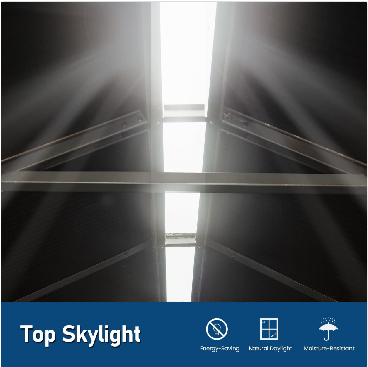
Image 5.1: The top skylight feature, designed to provide natural illumination within the shed, reducing energy consumption.
