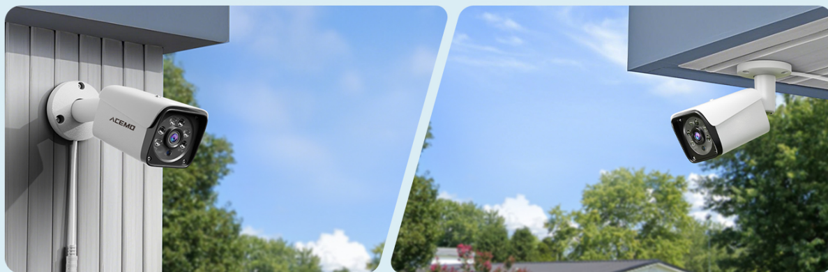
Figure 6: Examples of camera installation on both wall and ceiling surfaces.
