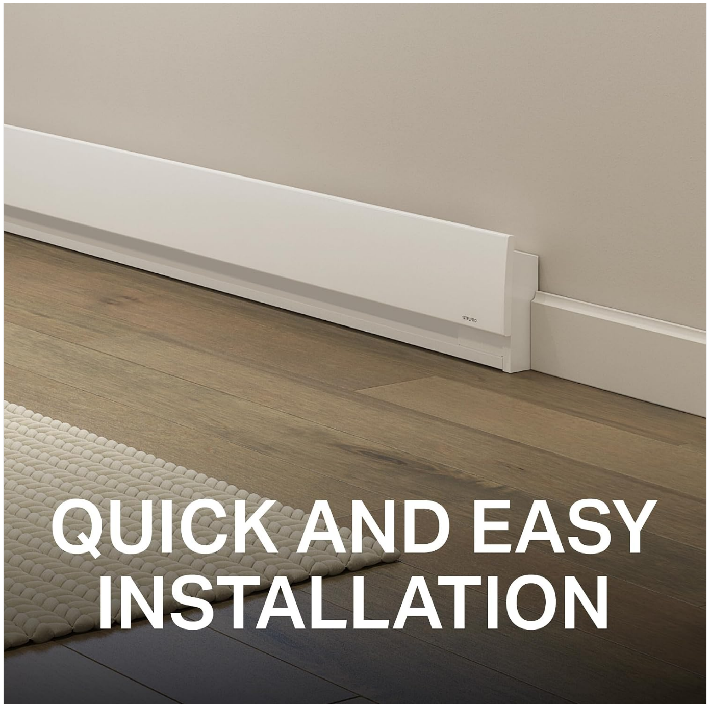
Figure 4.2: Example of a Stelpro baseboard heater installed in a living room, demonstrating its discreet placement.
