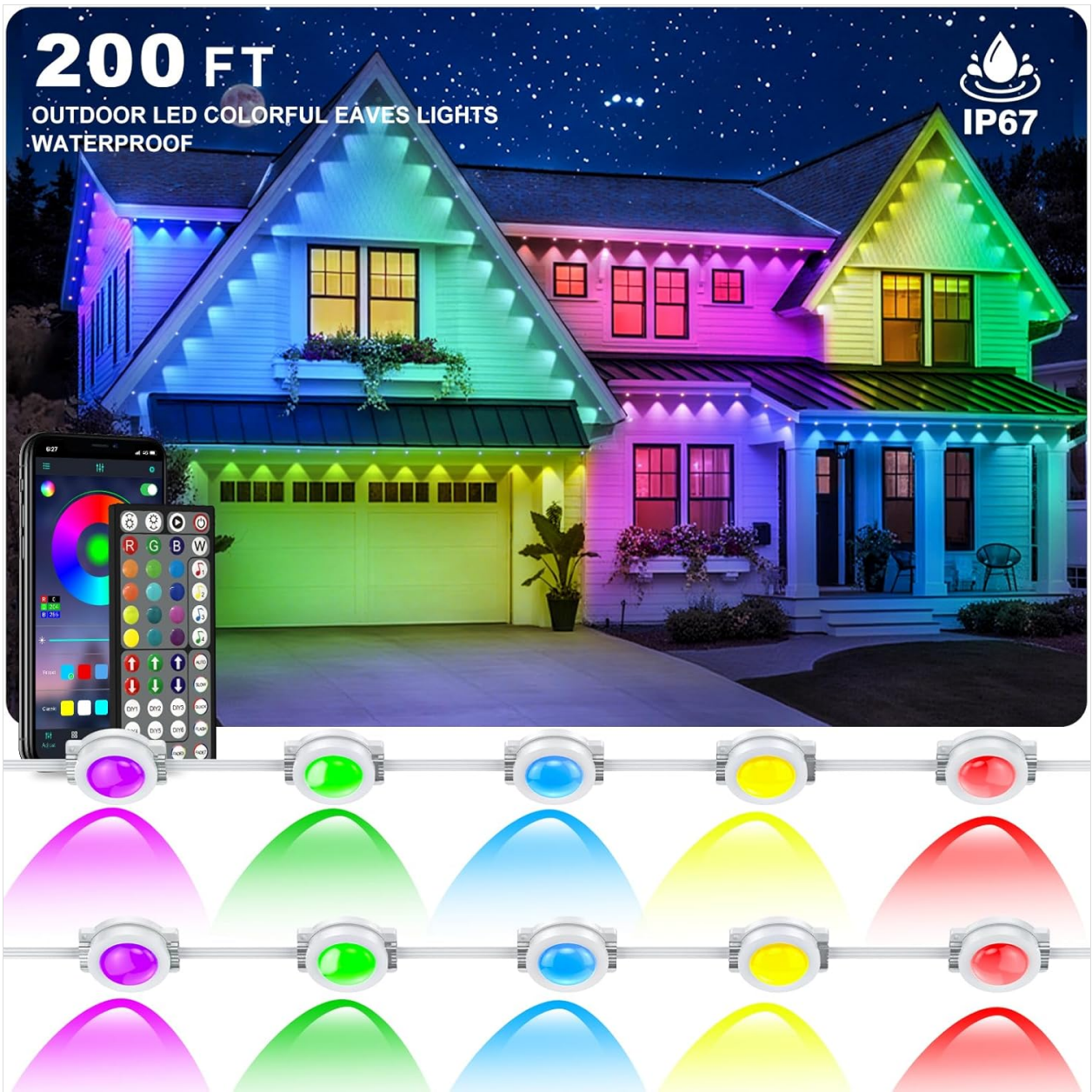
Image: An overview of the INZIDOL Eave Lights installed on a house, with an inset showing the smart app interface and the physical remote control for managing light settings.
