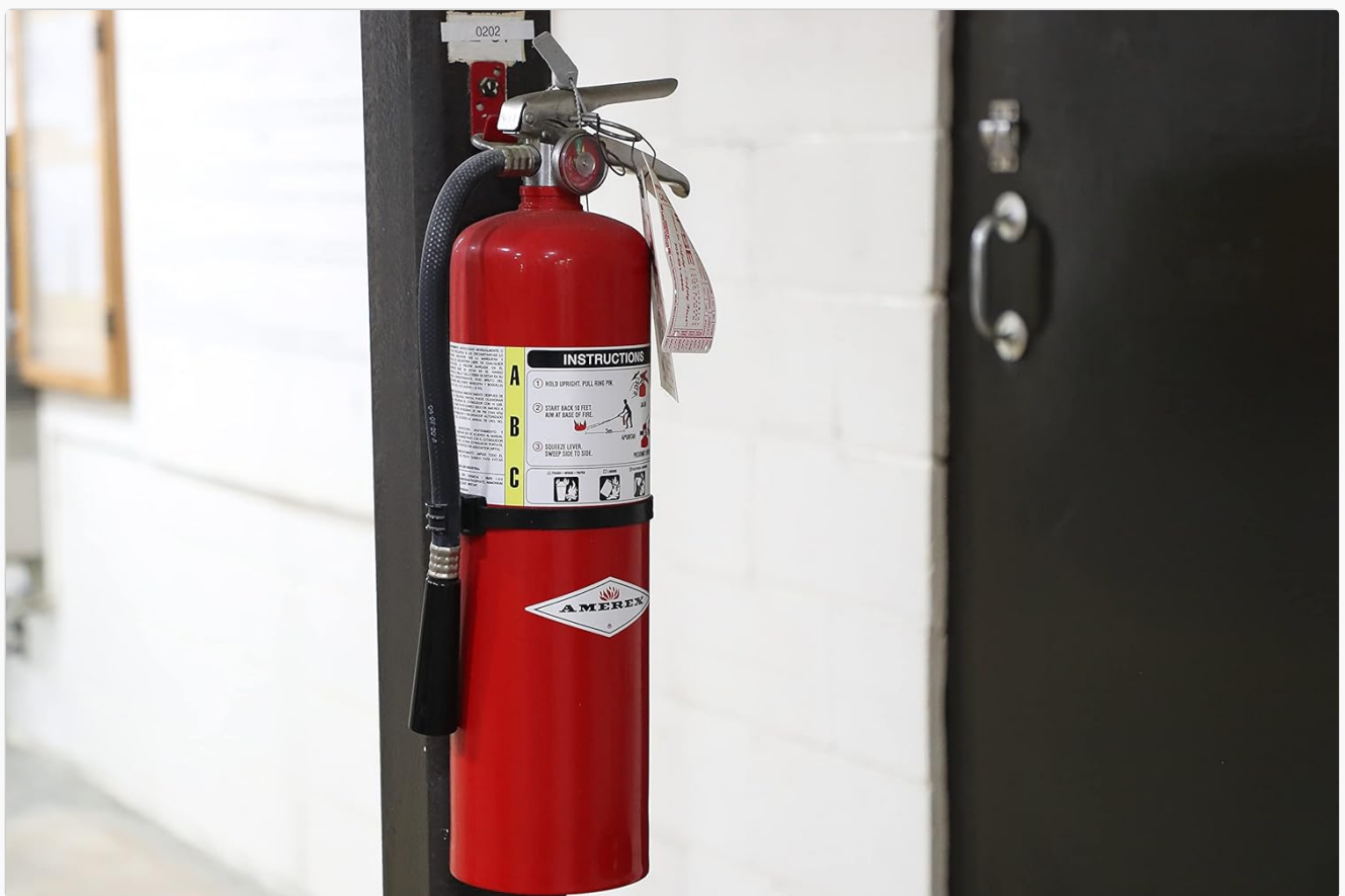
Figure 4: Mounted Extinguisher Close-up. A closer view of a mounted Amerex fire extinguisher, showing the bracket and the extinguisher's label clearly.
