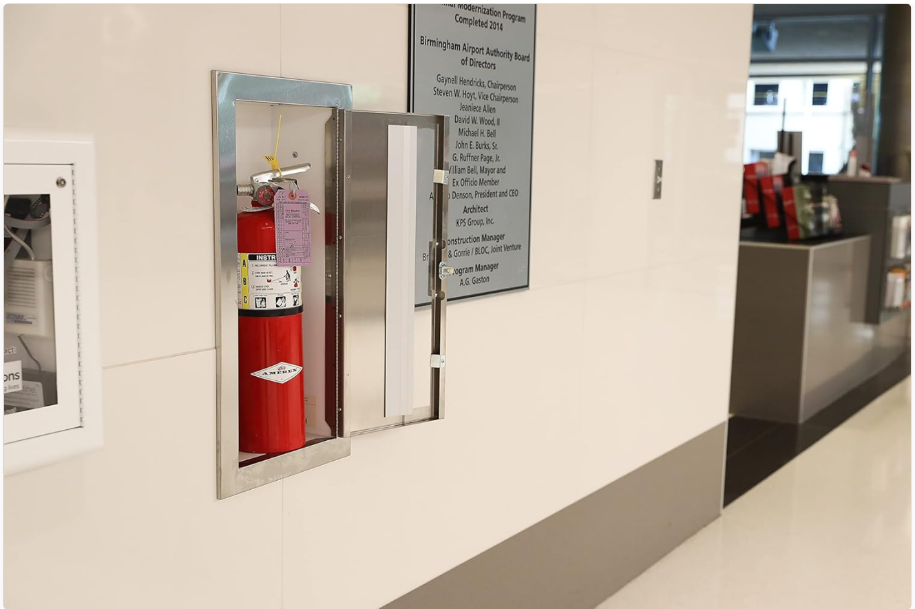
Figure 3: Extinguisher Mounted. This image shows an Amerex fire extinguisher securely mounted on a wall, demonstrating a typical installation scenario.
