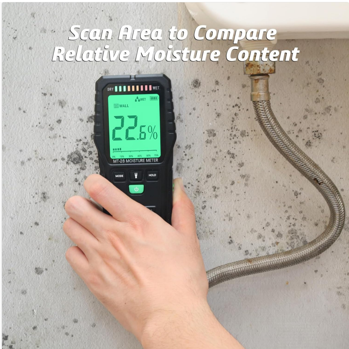
Figure 2: Scanning an area with the MT28 to compare relative moisture content on a wall.
