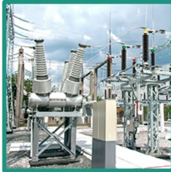
Image: Testing in power substations.
