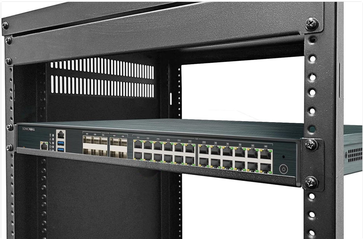
Figure 4: SonicWall NSA3800 appliance securely mounted in a server rack.
