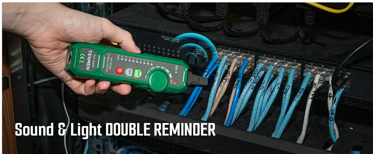
Image 6.2: Scanning cables connected to a PoE switch.
