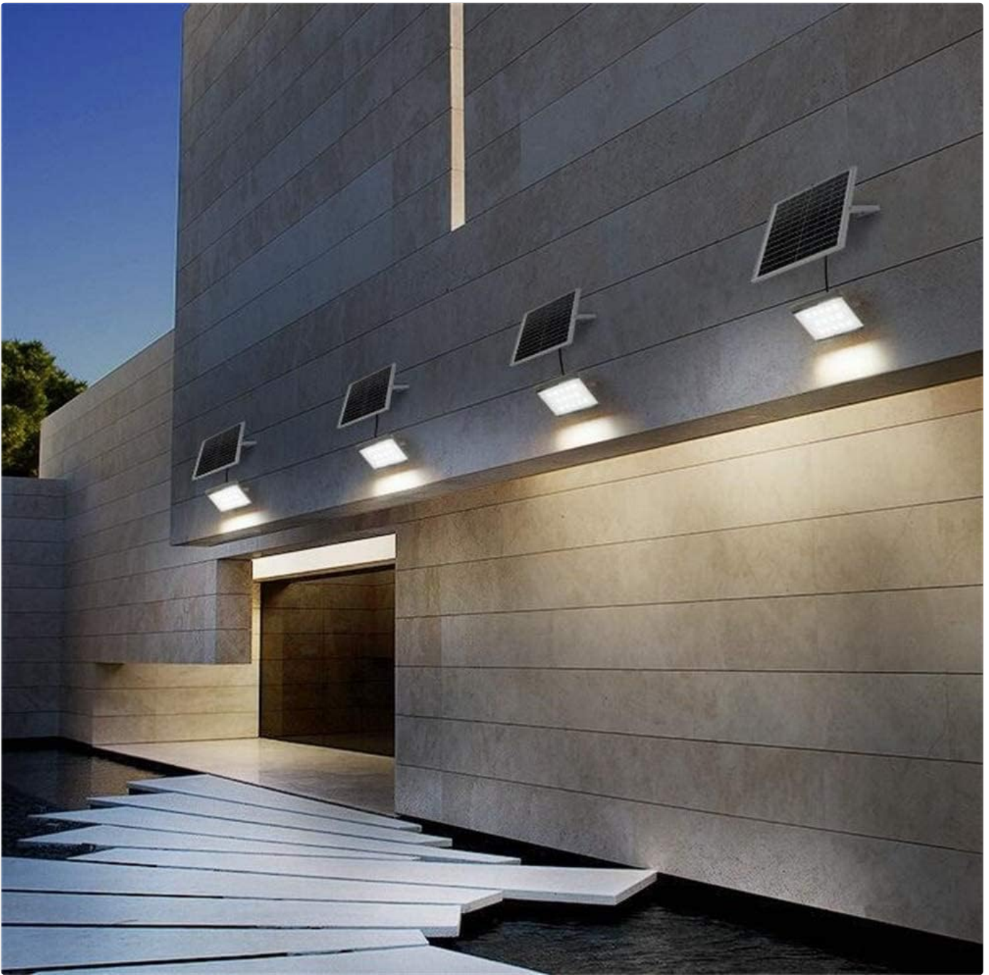
Image: Several solar floodlights mounted on the exterior wall of a modern building, demonstrating typical installation.
