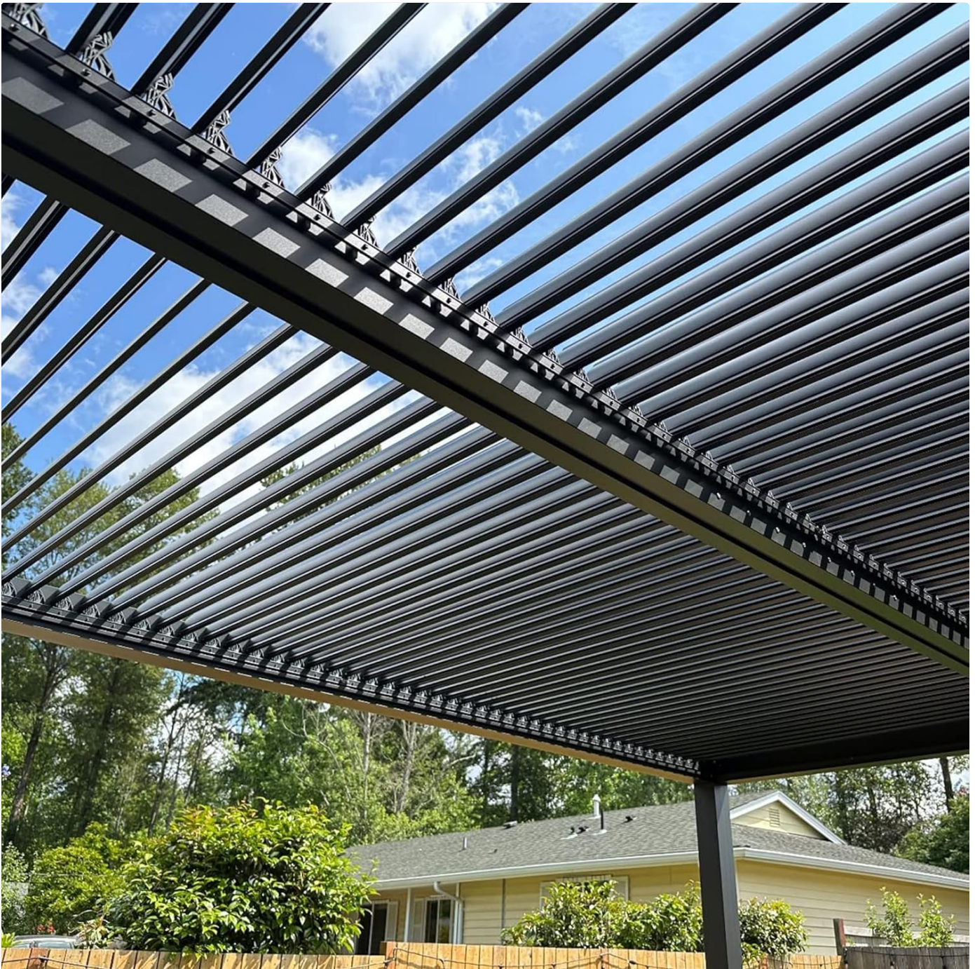
Figure 6: Louvers in an open position, allowing full sunlight.
