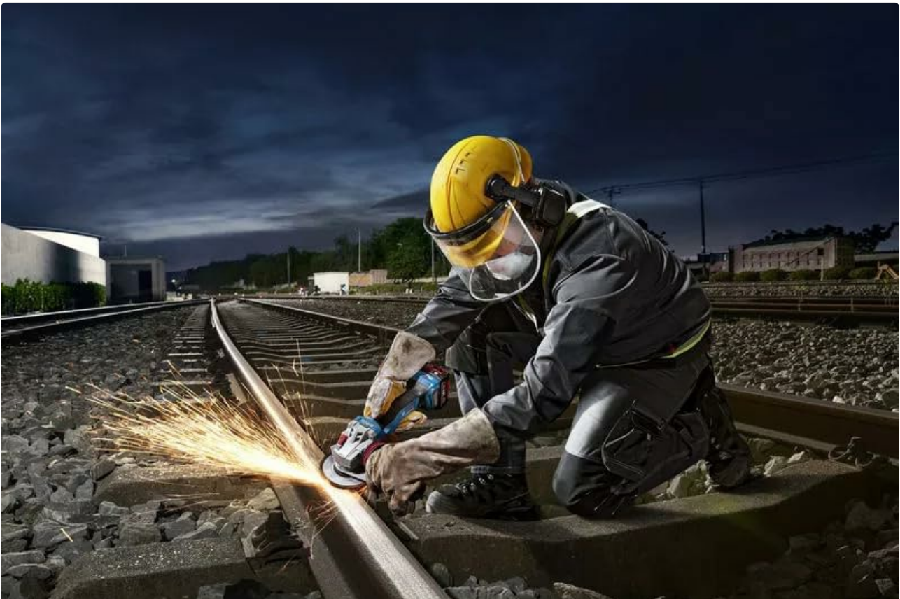
Image: A worker wearing safety gear, including a hard hat and face shield, using the BOSCH GWS 18V-11 S angle grinder to cut a metal component on a railway track, generating sparks.
