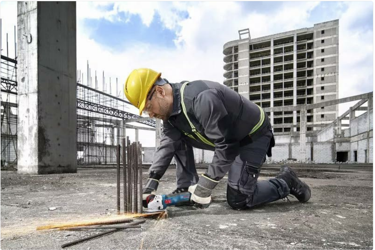
Image: A worker in safety attire using the BOSCH GWS 18V-11 S angle grinder to cut rebar on a concrete surface at a construction site, with sparks visible.
