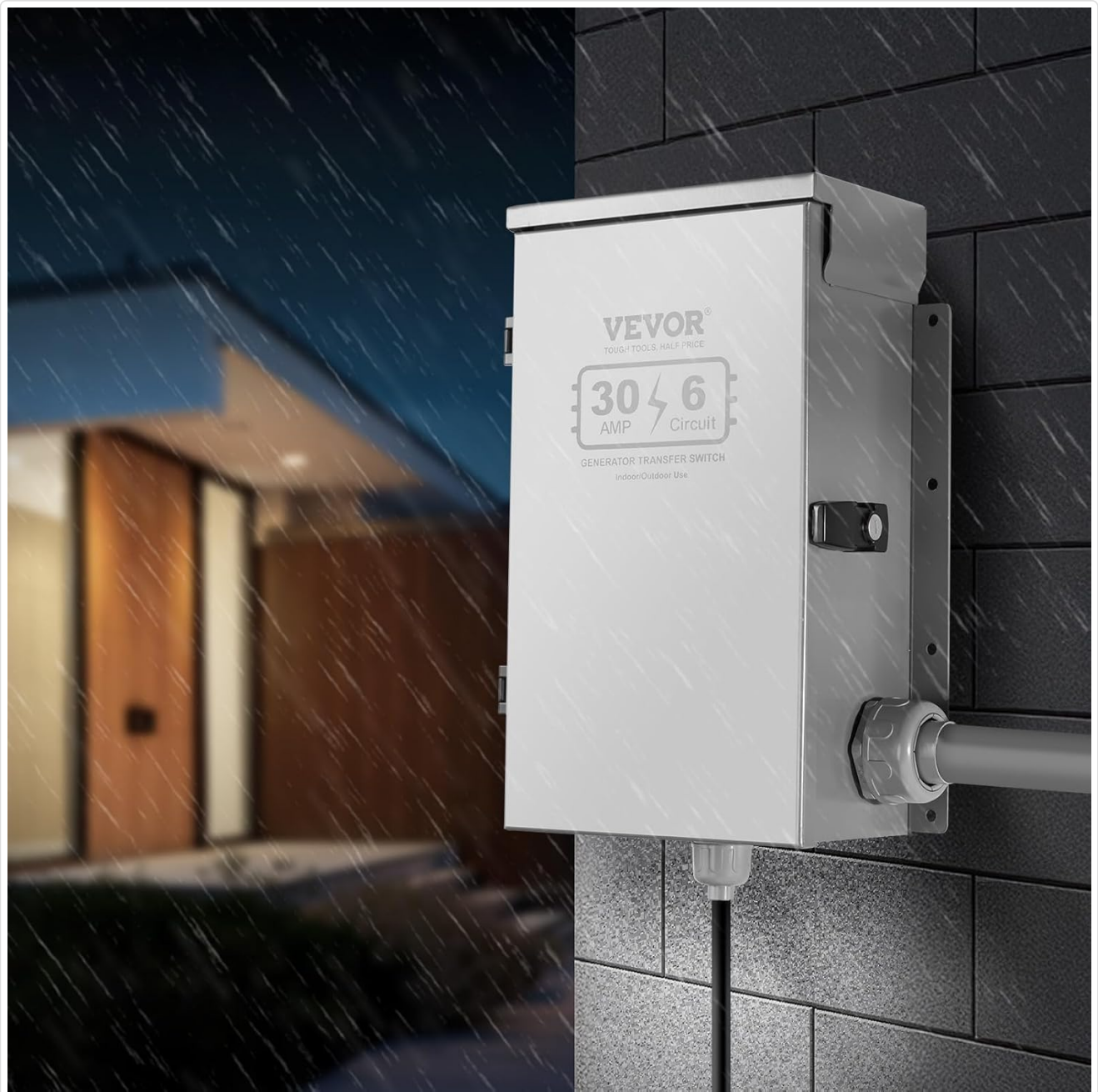
Image: The VEVOR transfer switch installed on an exterior wall, demonstrating its NEMA 3R weatherproof design in a simulated rainy environment.
