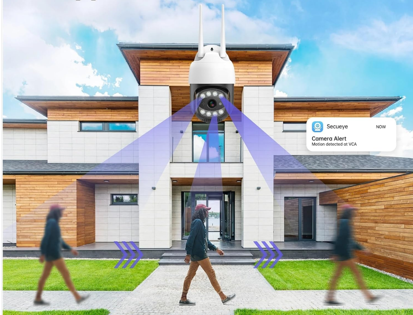
Figure 4.1: Camera physical installation and pan-tilt range. The camera can pan 330 degrees and tilt 90 degrees, allowing for extensive coverage.
