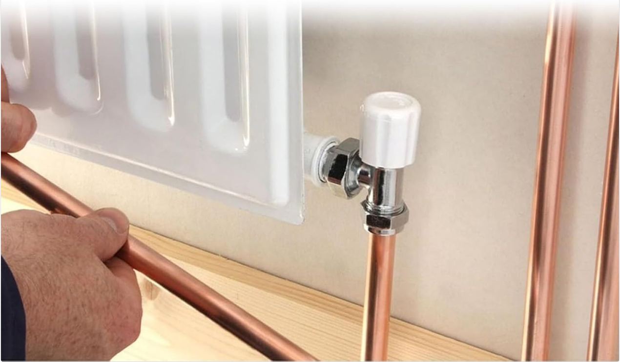
Image 6: Visual comparison showing a flattened copper tube and a tube successfully rounded using the tool, demonstrating the repair capability.
