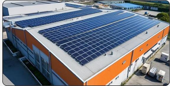
Solar Power Plant System
