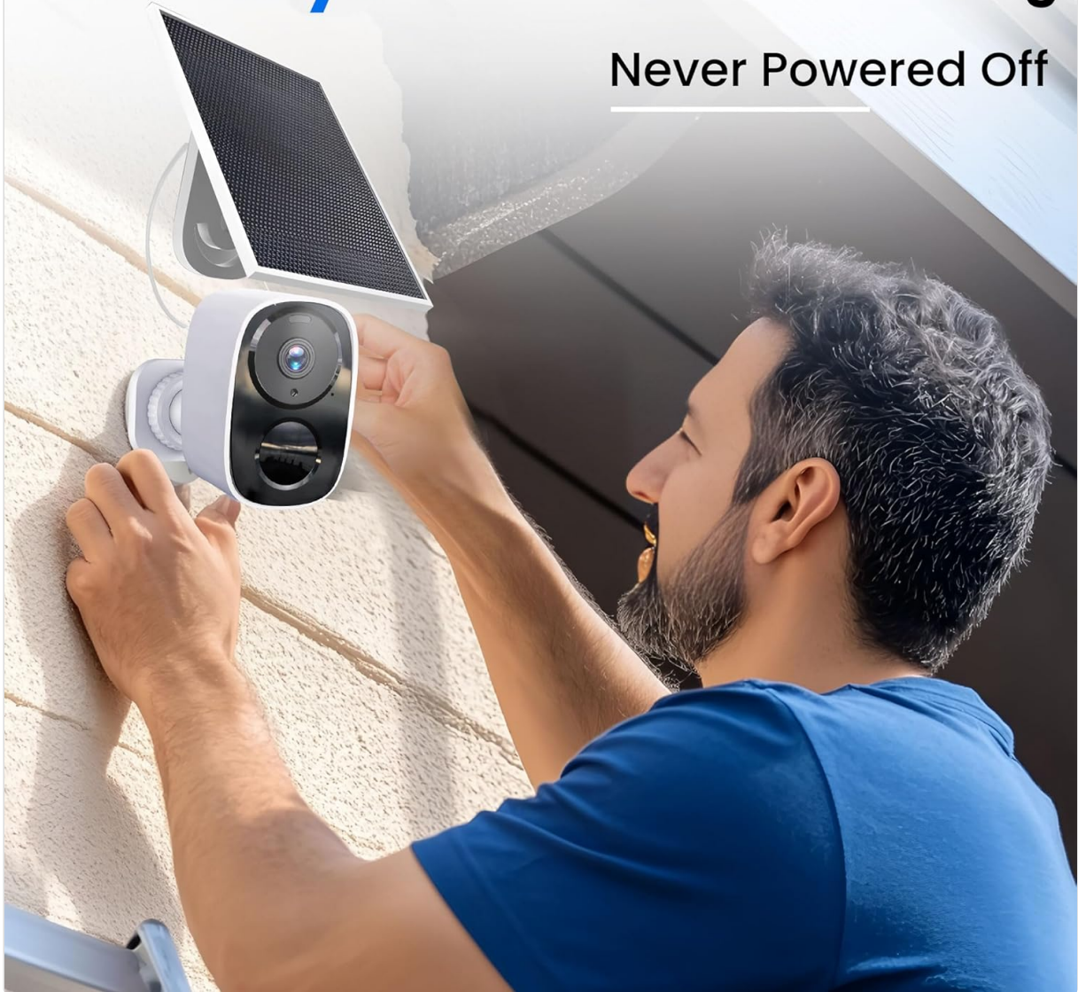
Image 4.1: Installation of the HITELLARCAM CB54. This image shows a person installing the camera and solar panel on an exterior wall, demonstrating the mounting process.
