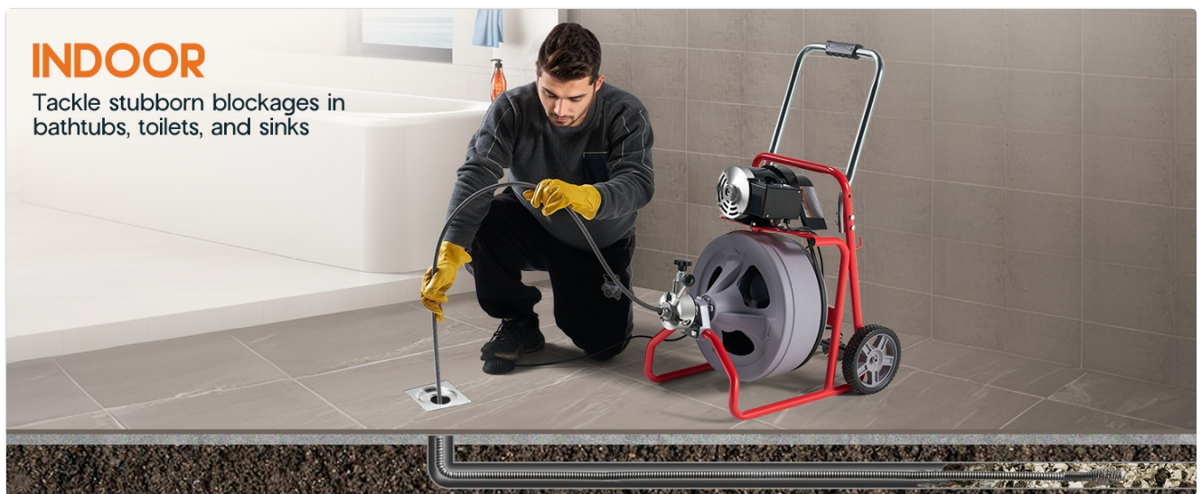
Figure 5.4: Tackling indoor blockages.
