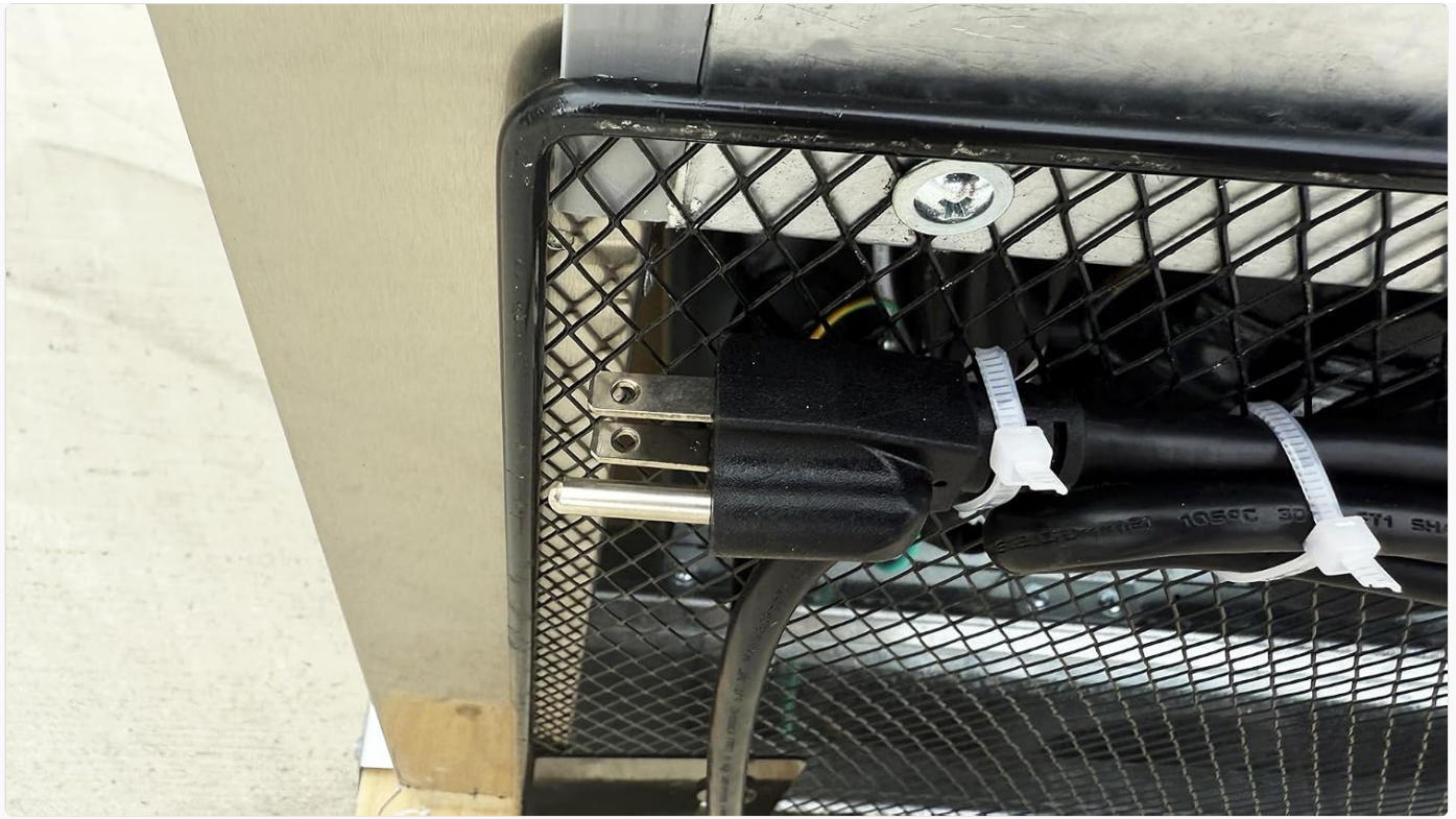
Figure 3: Power cord and plug connection point.
