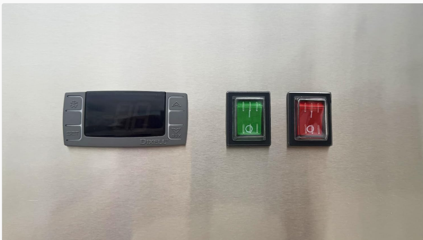
Figure 5: Digital temperature controller and main power switches.
