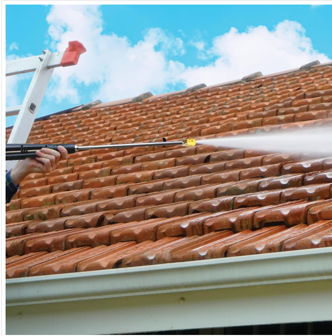
Figure 4.2: Demonstrating the pressure washer's capability for cleaning outdoor surfaces such as tiled roofs.
