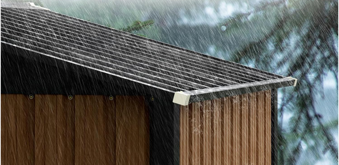
Image 7.1: The shed's roof during rainfall, illustrating its design for protection against weather elements.
