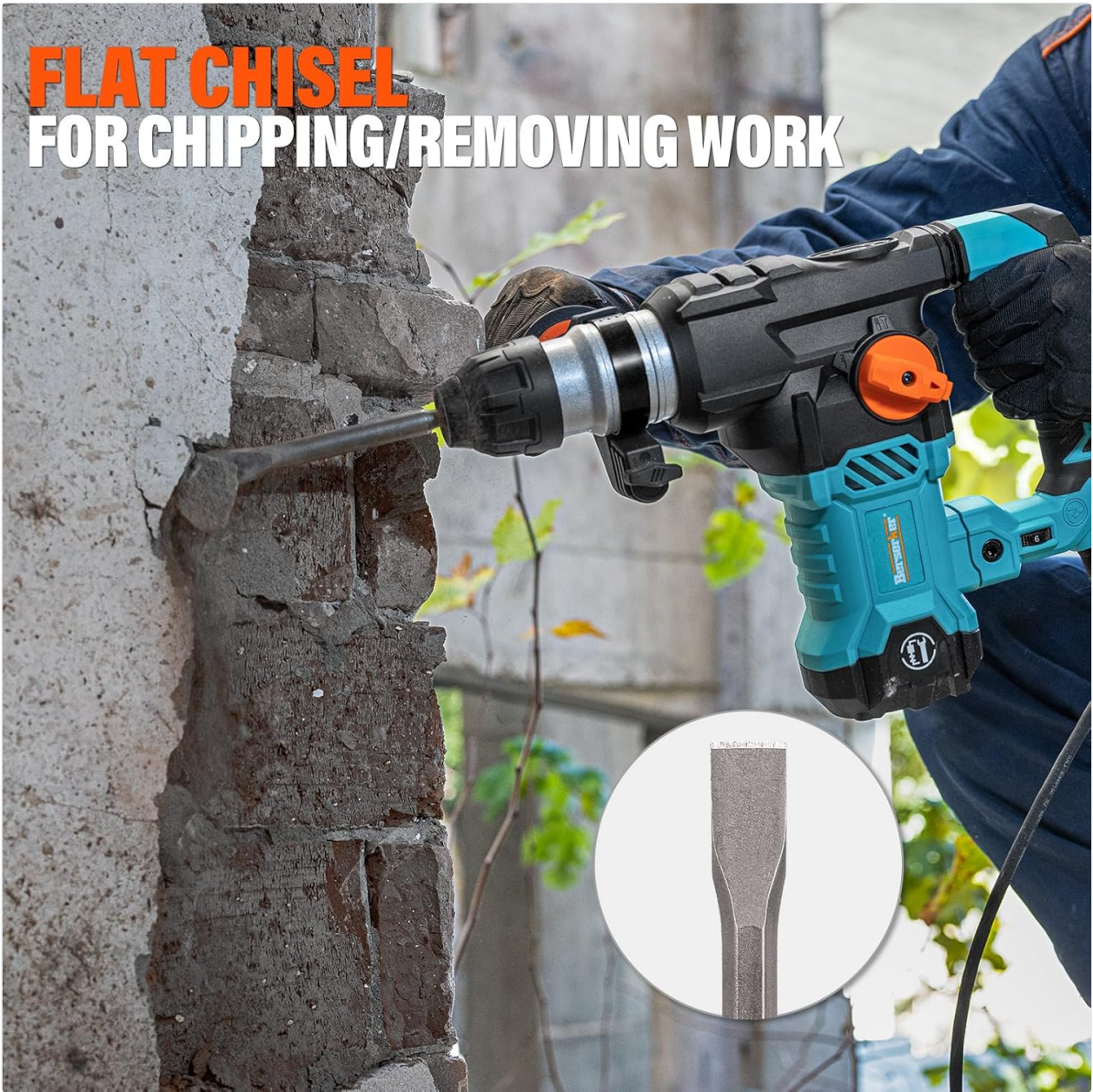
Image 5.2: A flat chisel being used with a rotary hammer for chipping and material removal work.
