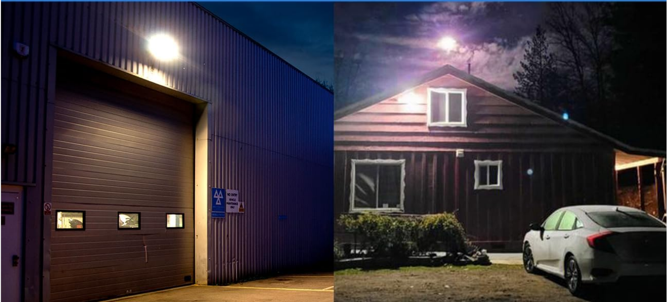
Figure 4.1: Example of installed solar street lights providing bright illumination for a garage and surrounding area.
