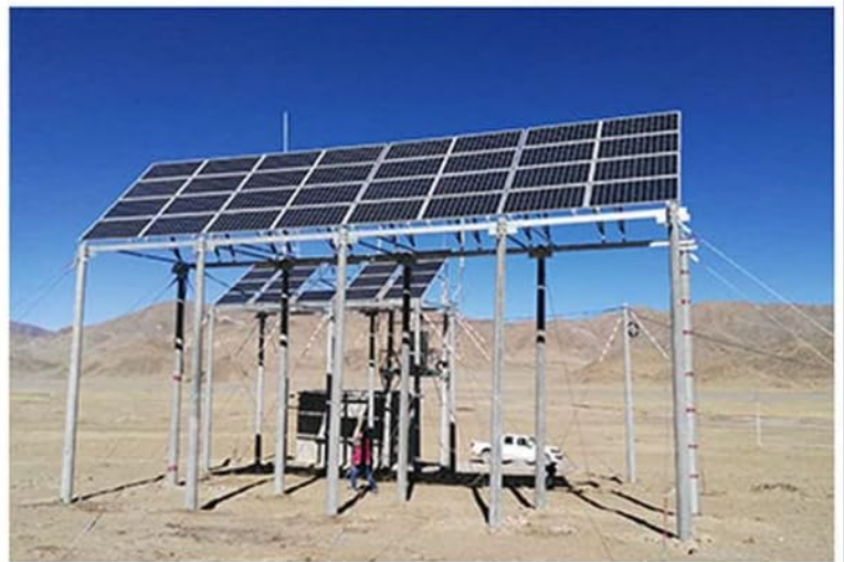
Power station system
