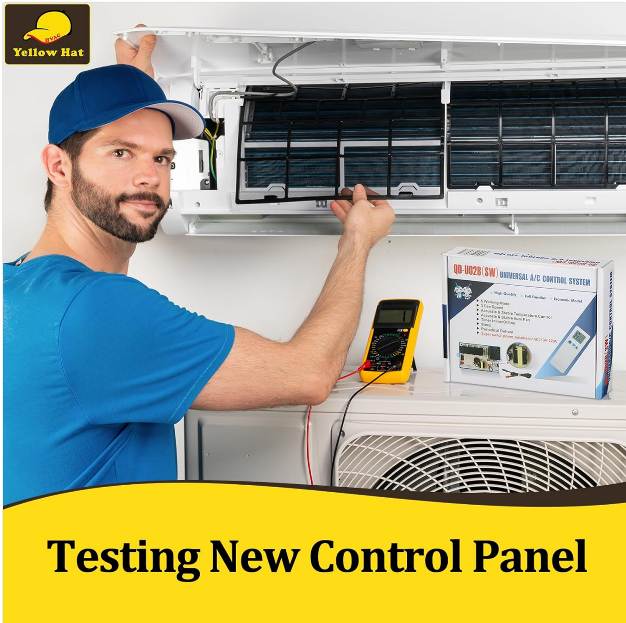
Image 4.3: A technician using a multimeter to test the functionality of a newly installed control panel in an AC unit.
