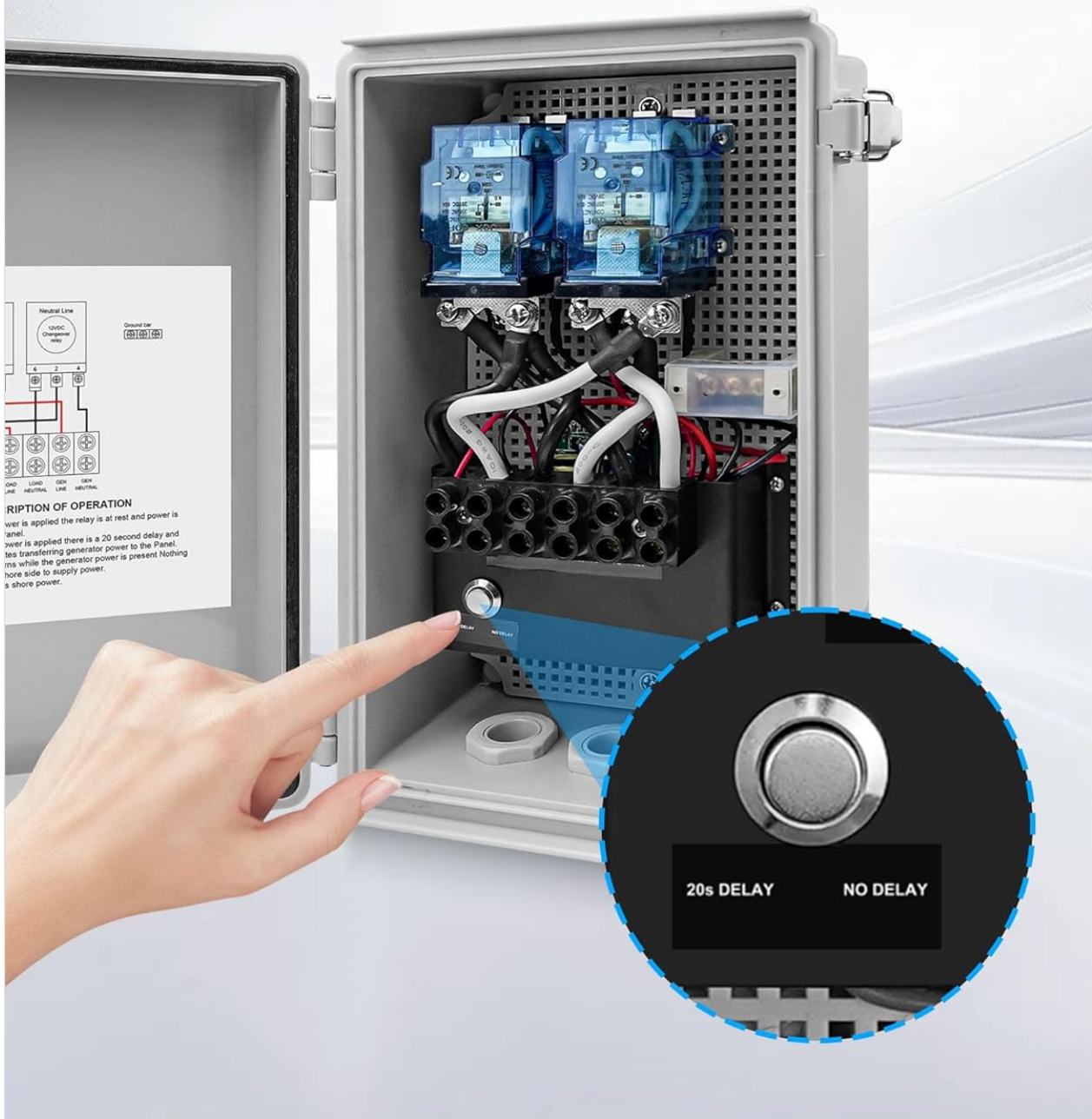
Figure 3.3: Detail of the 20-second delayed start mechanism, which ensures voltage stability before power transmission.
