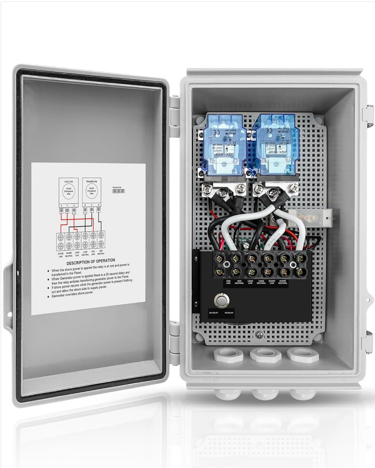
Figure 3.1: Internal components and basic wiring layout of the transfer switch. This view illustrates the relays and terminal
