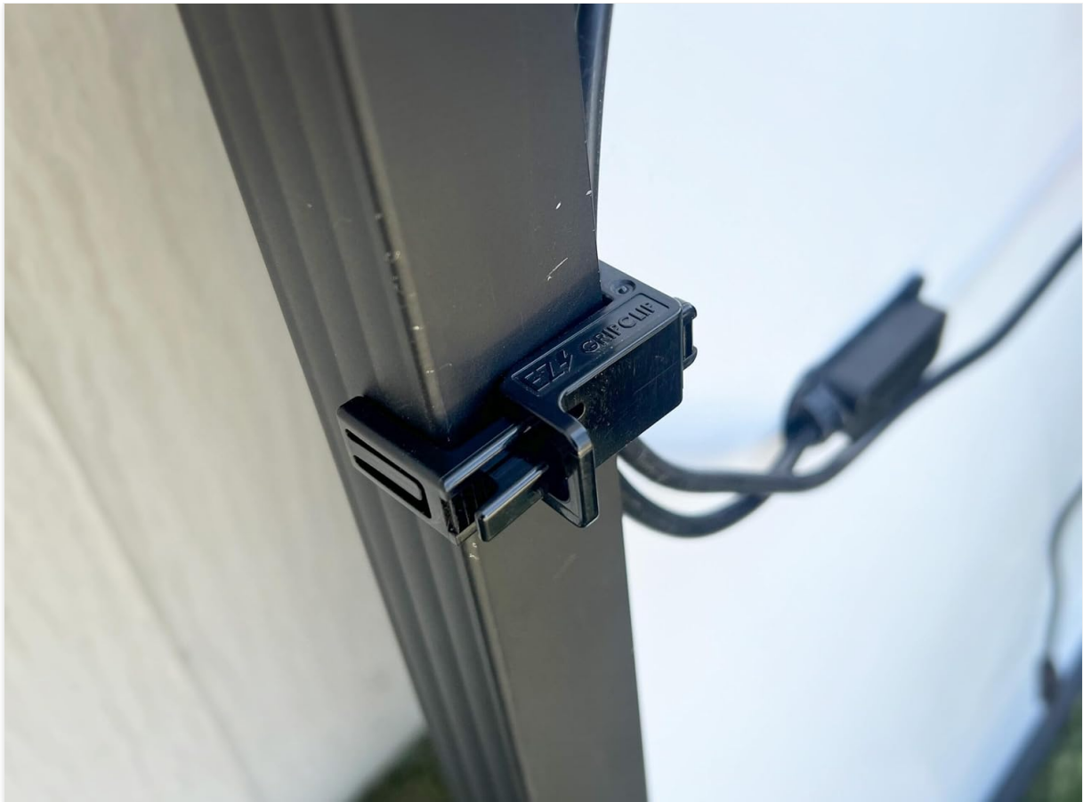
Figure 2: The EZ Solar GripClip in use, attached to a black vertical frame, likely a solar panel support. Two black electrical wires are neatly routed and secured by the clip, demonstrating its function in wire management.
