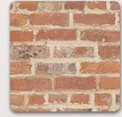
Brick Wall (Need anchors)
