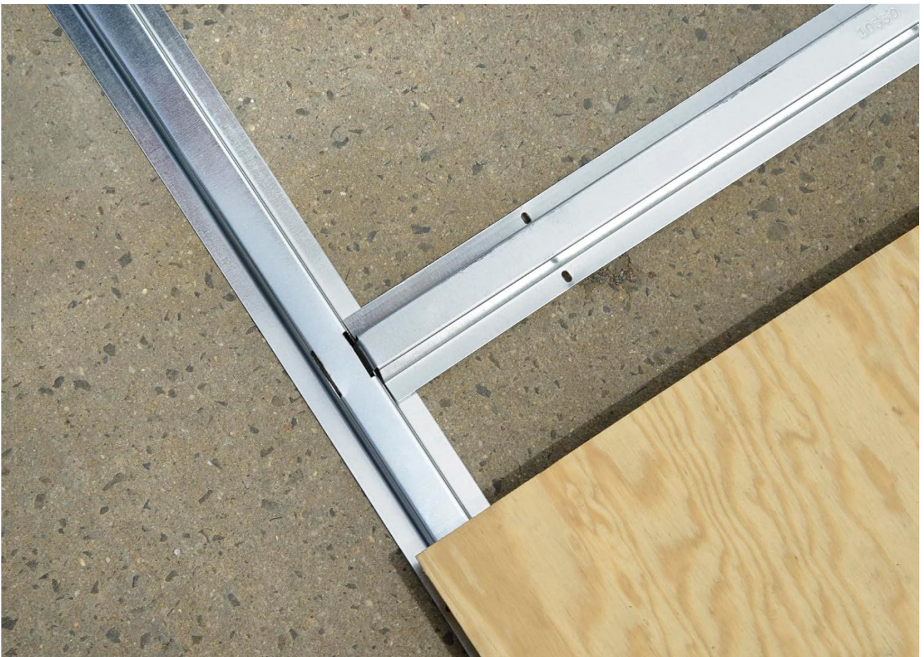
Figure 5.4: A close-up image focusing on a corner section where the plywood flooring meets the metal frame. This highlights how the flooring material integrates with the frame structure.
