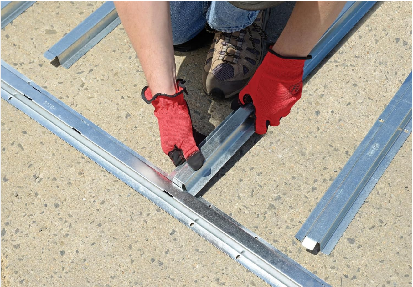
Figure 5.1: A close-up view of an individual wearing red work gloves, demonstrating the process of connecting two metal frame components. This illustrates the initial assembly of the floor frame structure.
