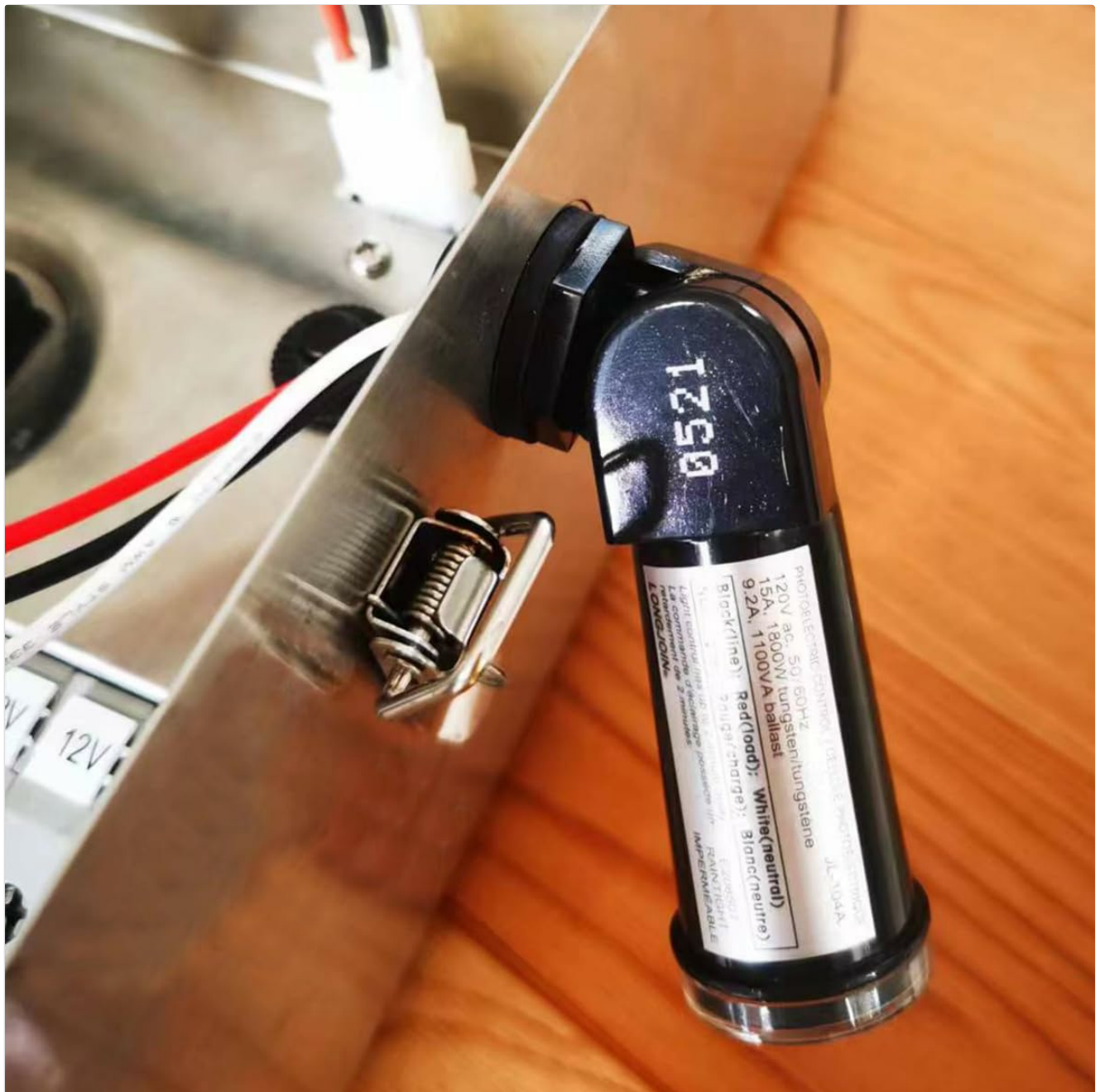
Image Description: A detailed close-up of the photocell sensor, highlighting its connection to the transformer casing. The sensor's cylindrical body and mounting mechanism are clearly visible.
