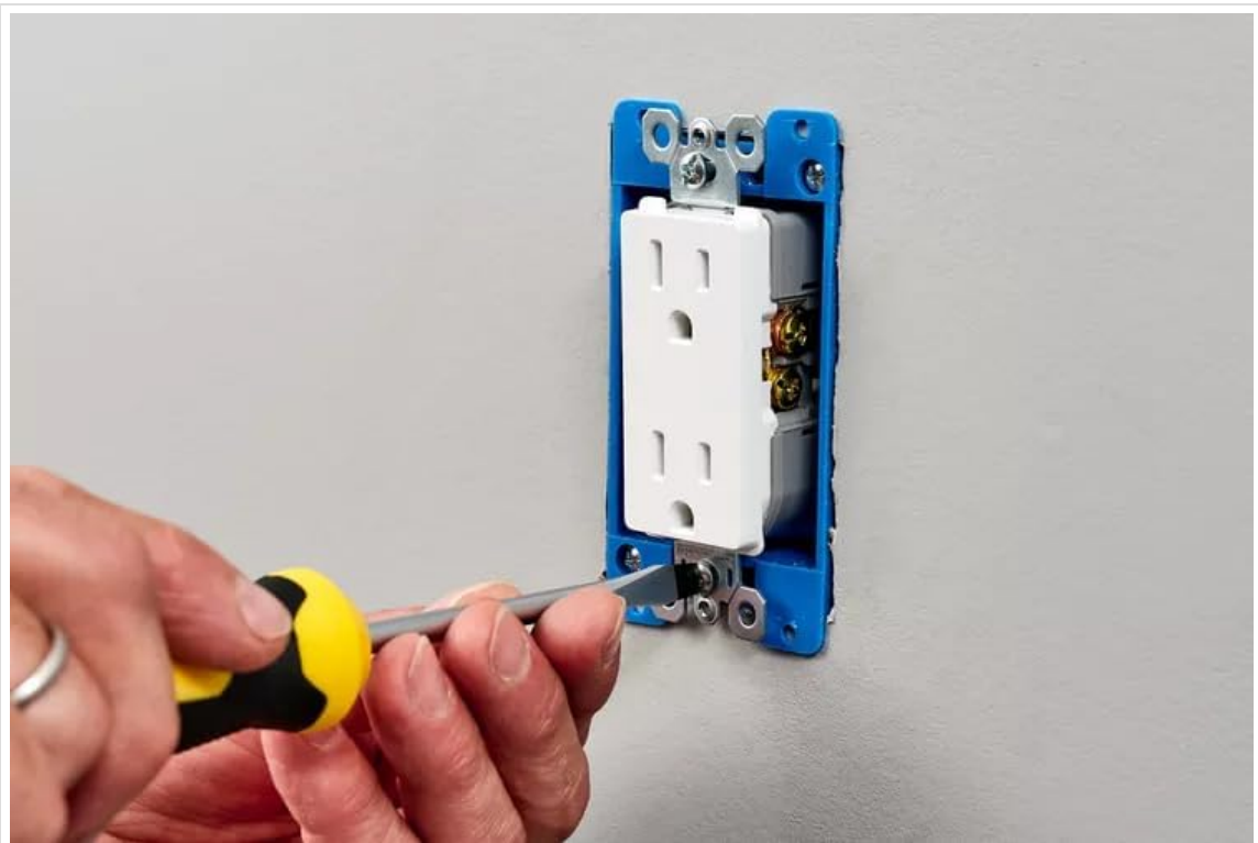
Figure 5.2: Securing the wall outlet camera into an electrical wall box using a screwdriver.
