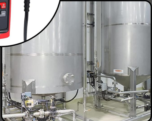
Oil storage tanks
