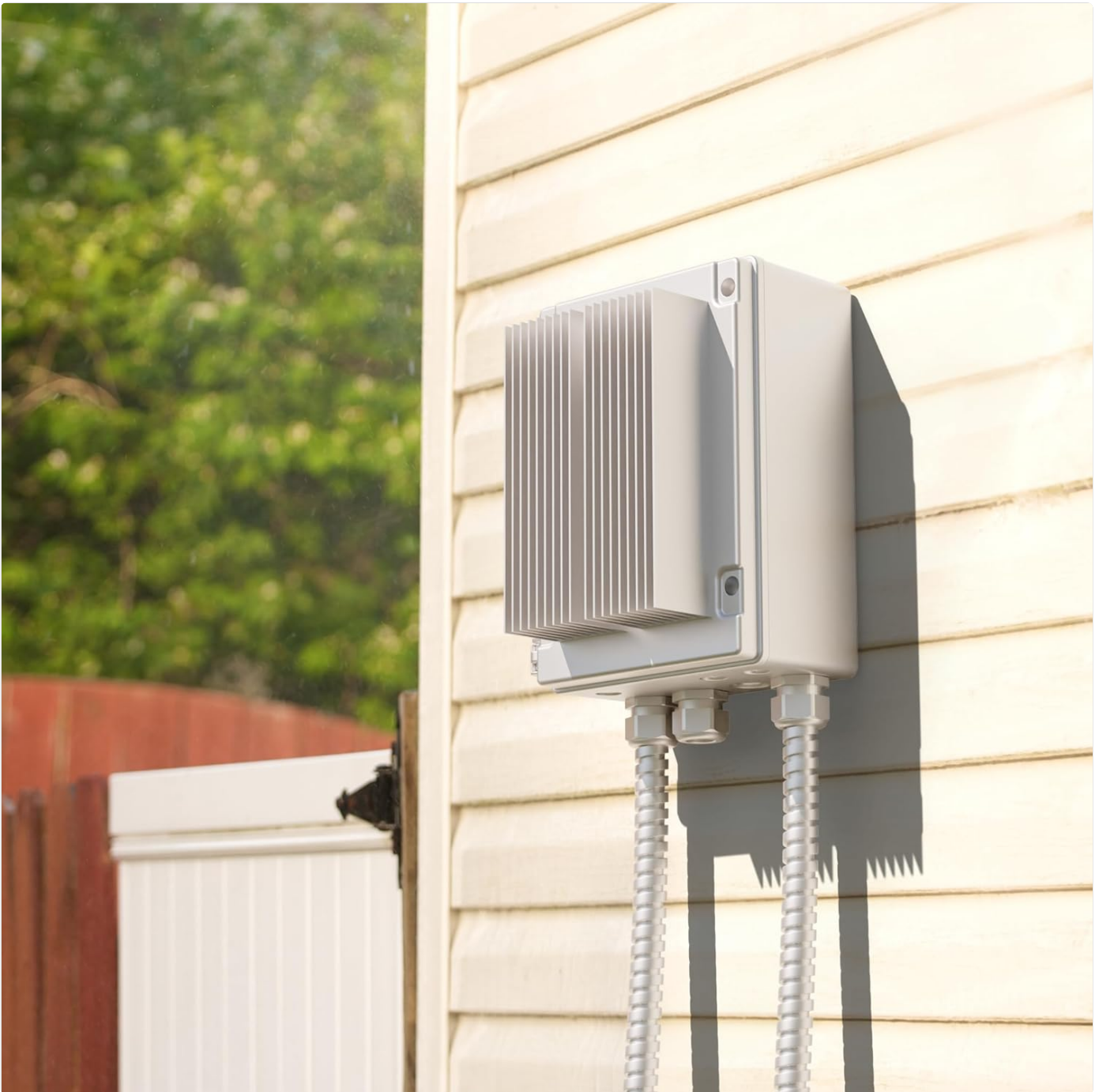
Figure 2: Example of the controller mounted on an exterior wall with conduit connections.
