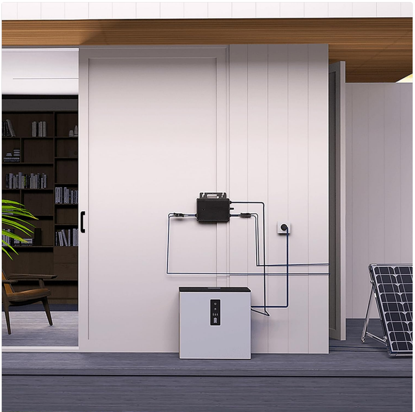
Figure 2.3: Example of an outdoor installation setup for the MS-A2 battery system.
