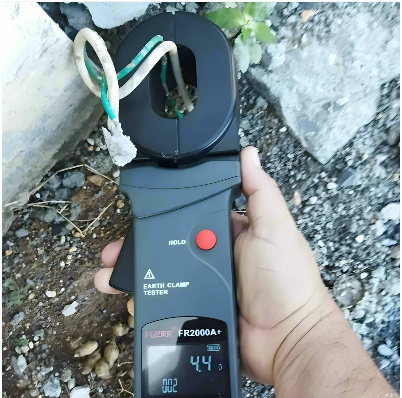
Figure 3: The FR2000A+ clamp earth resistance tester in use, measuring resistance by clamping around a grounding wire.
