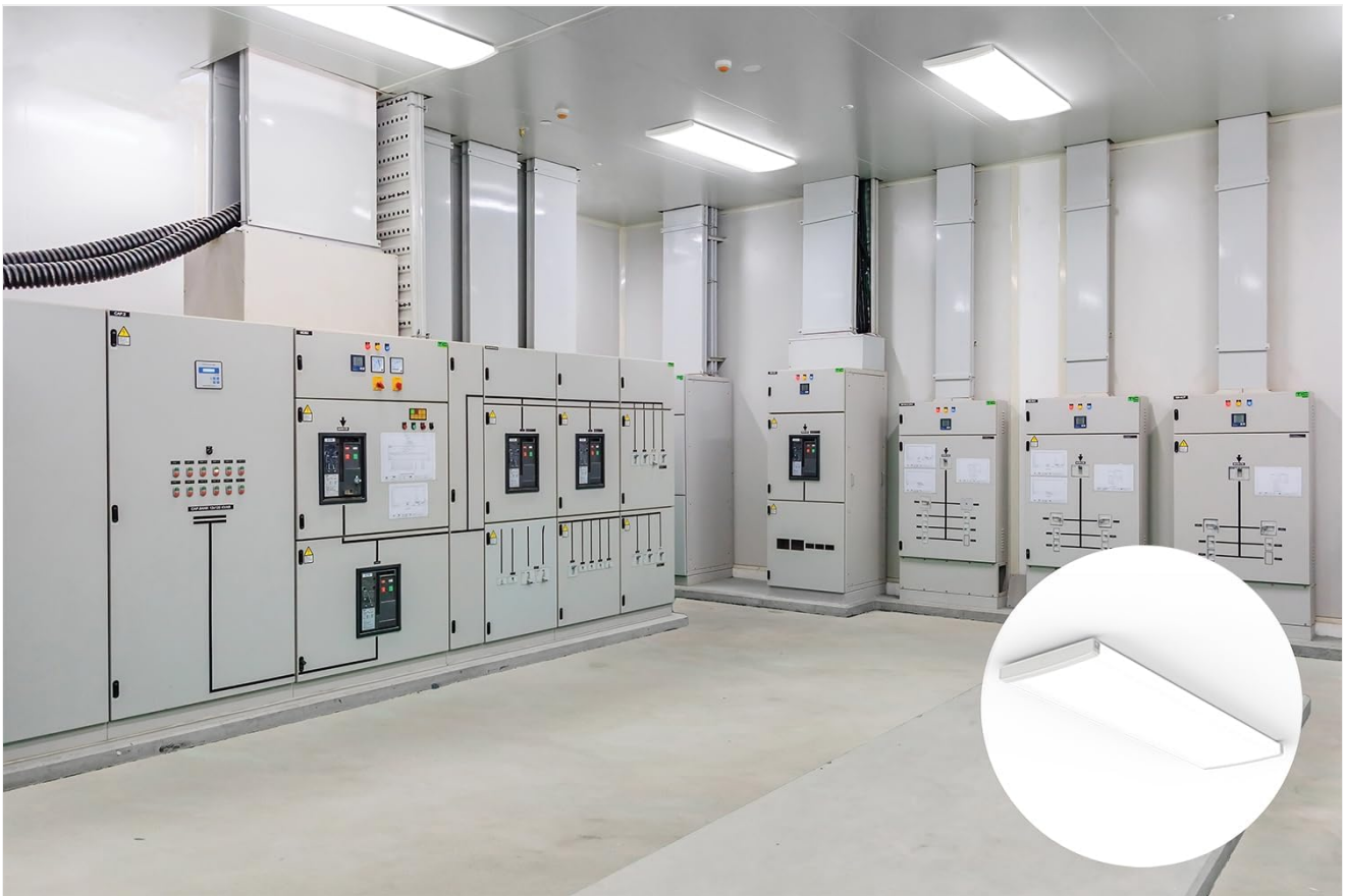
Image 10.3: TruWrap fixture installed in a utility room.
