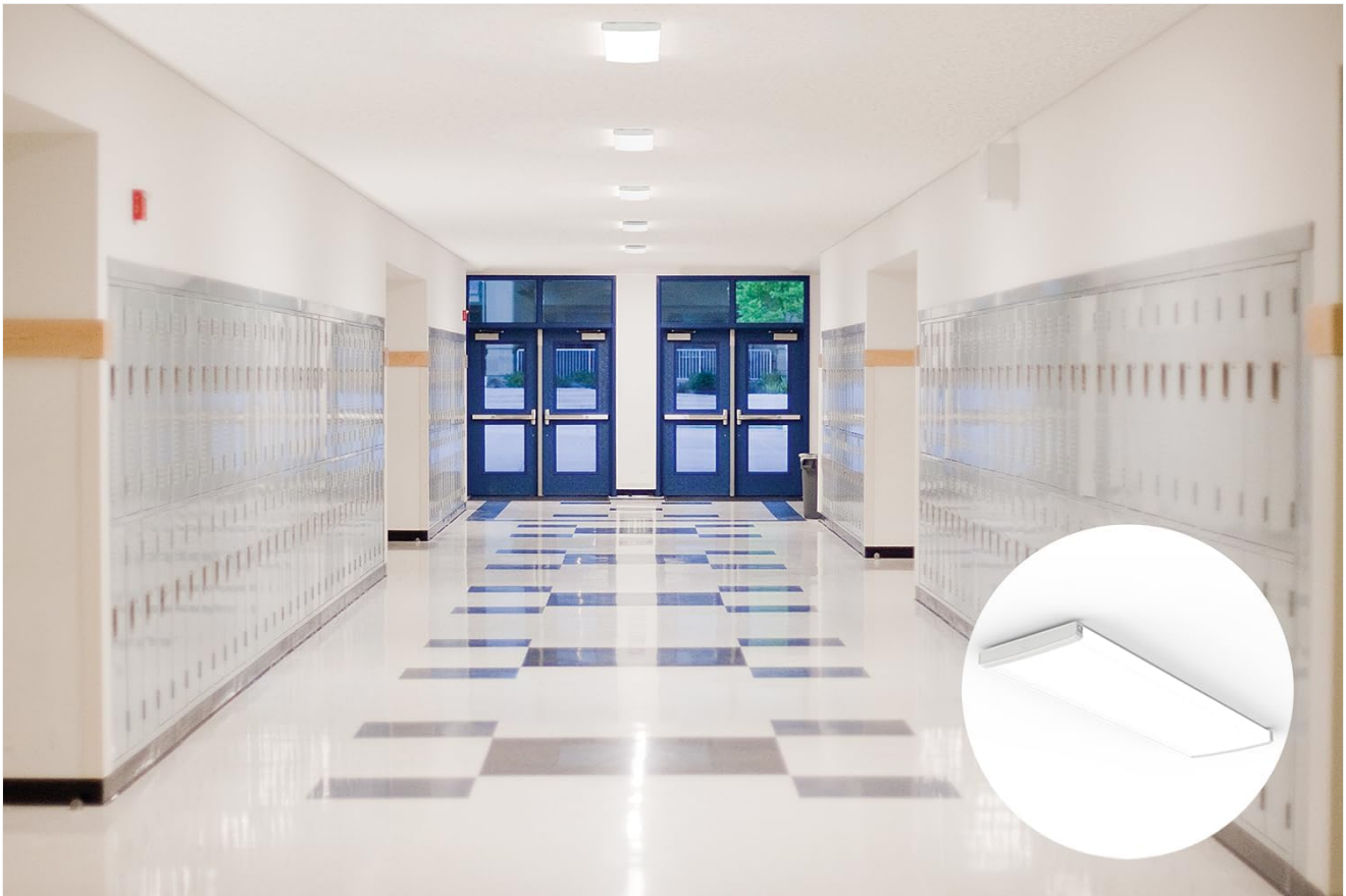
Image 10.2: TruWrap fixture installed in a hallway.
