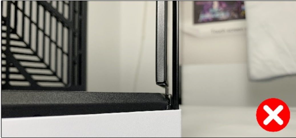
Incorrect installation: Monitor not fully inserted, causing it to dangle.
