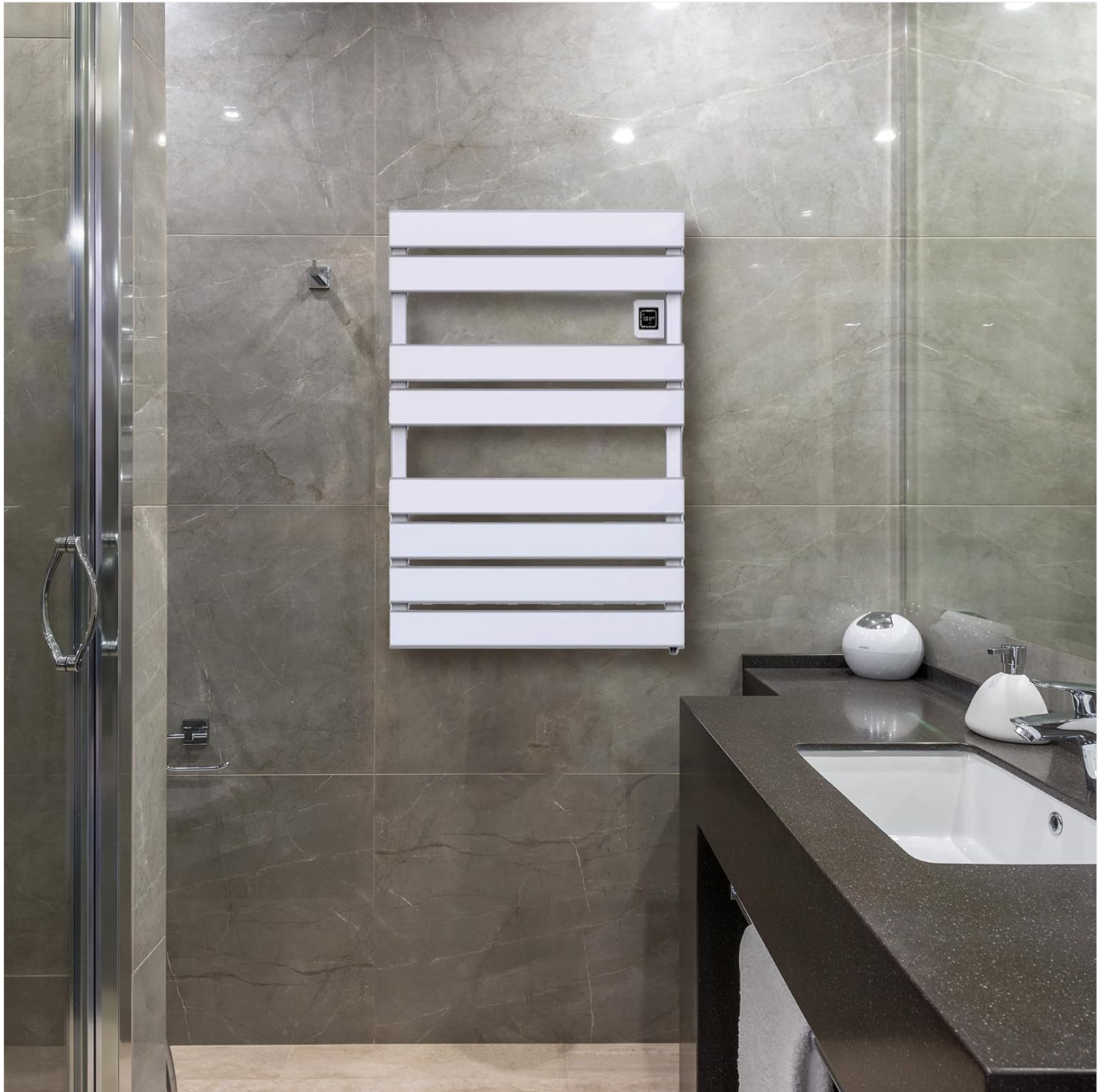
Figure 3: Example of the towel dryer installed in a bathroom setting.
