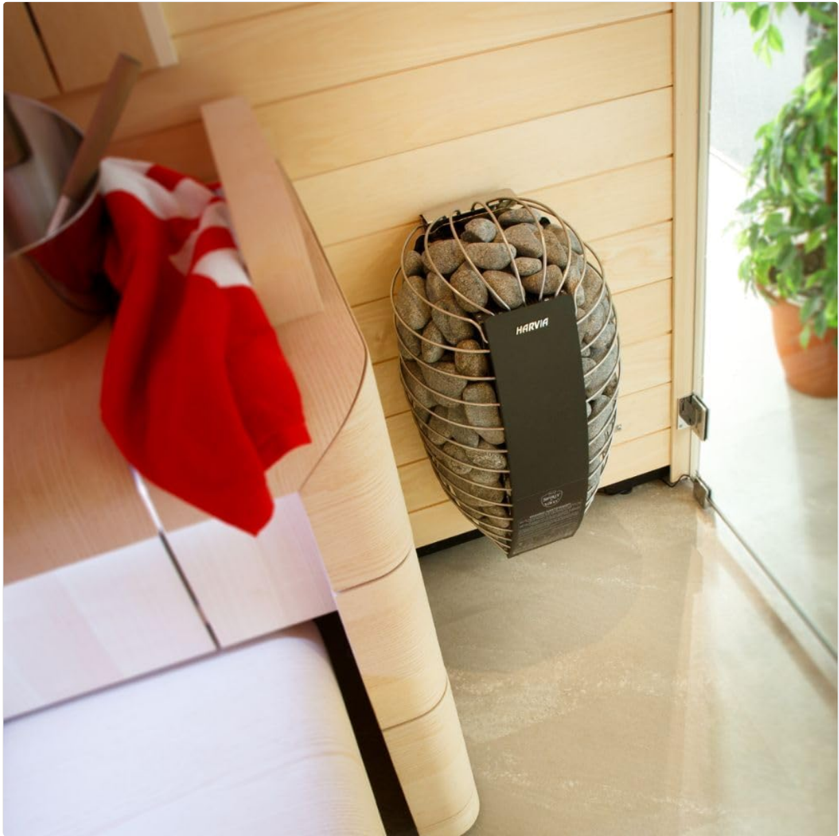
Image: The Harvia Spirit SPE Sauna Heater seamlessly integrated into a wooden sauna, demonstrating its wall-mounted installation.
