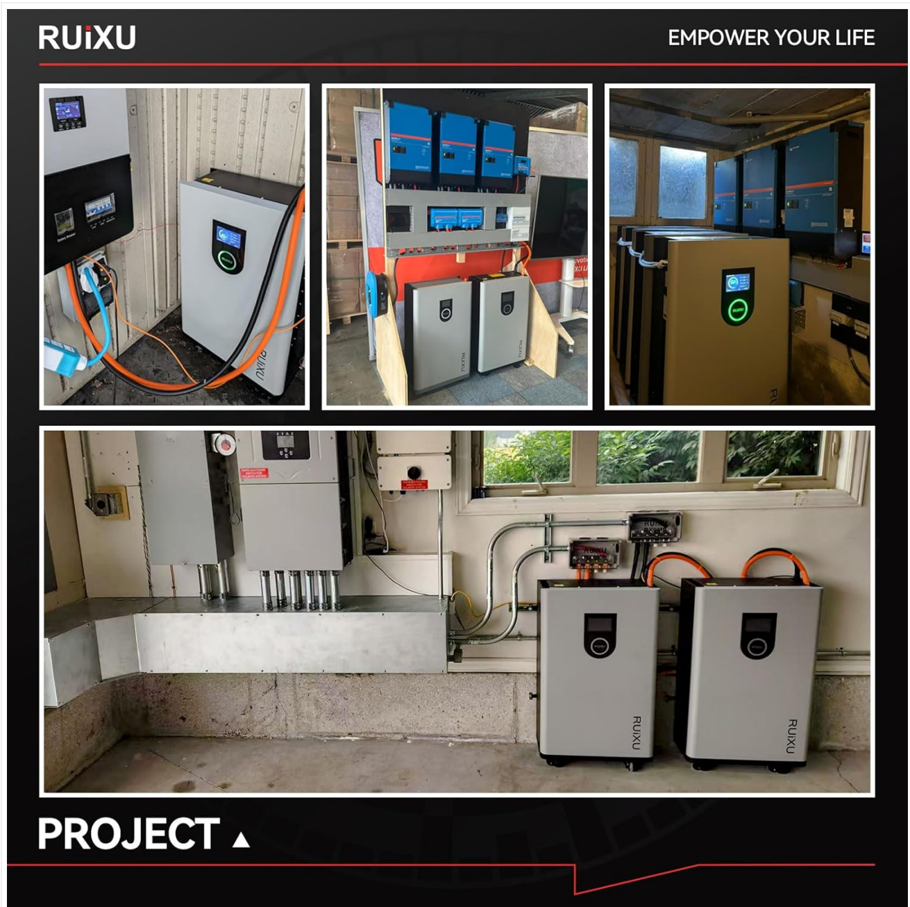
Figure 4.1: This image displays several real-world installations of the RUIXU Lithi2-16 battery, demonstrating its versatility in different energy storage projects, including single and multiple unit setups.
