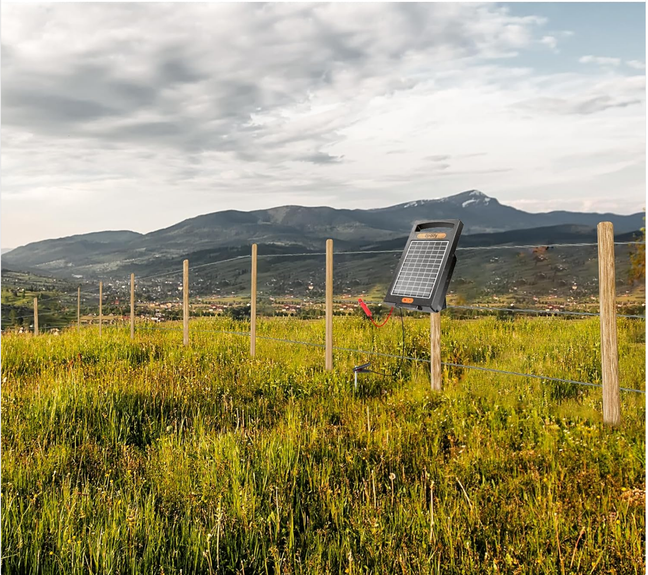
Image 5.2: The solar fence charger installed on a post, connected to an electric fence line and a ground rod, providing protection over a wide area.
