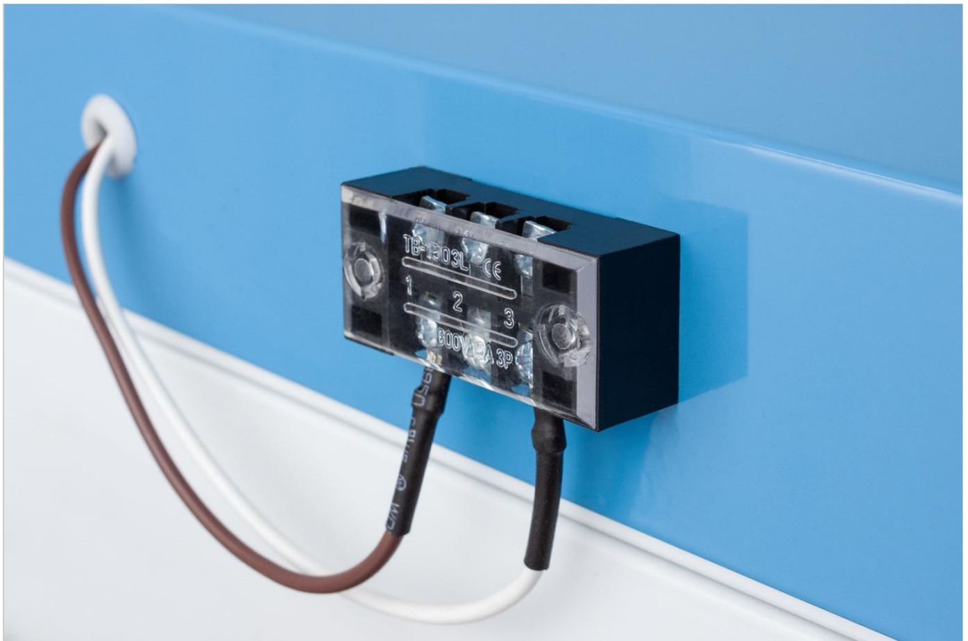
Figure 2: Remote alarm contacts for external monitoring integration. Wires are connected to a terminal block.
