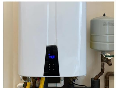
GAS WATER HEATER
