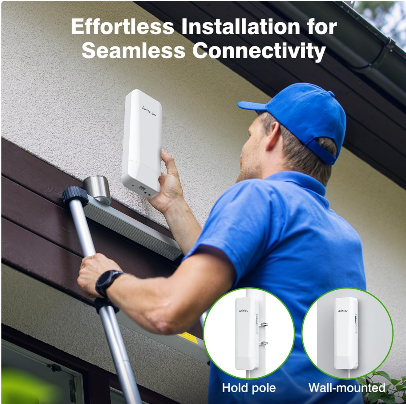
Image: A person installing an Adalov CPE368 Wireless Bridge on the exterior wall of a building, demonstrating wall-mounted installation.
