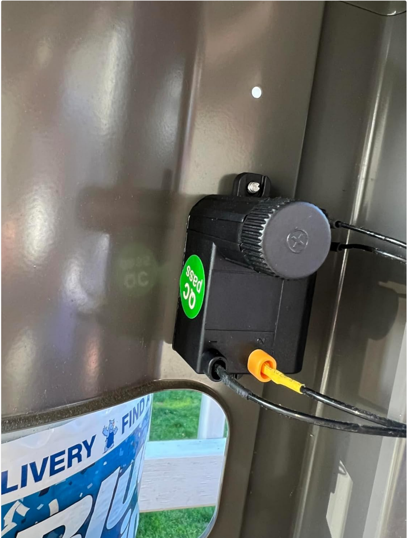
Figure 5.2: The MCAMPAS igniter module securely installed inside the grill cabinet. The module is attached to the inner wall, and its wires are connected, demonstrating a proper installation.
