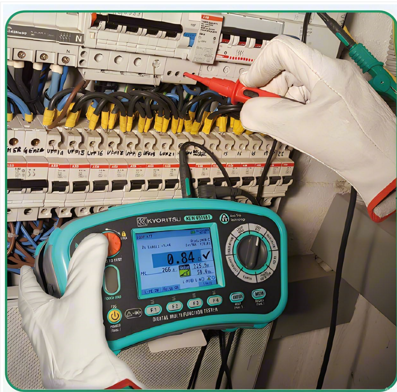
Figure 4.2: KYORITSU KEW 6516 Multi Function Tester in use, performing an electrical measurement within a circuit breaker panel.
