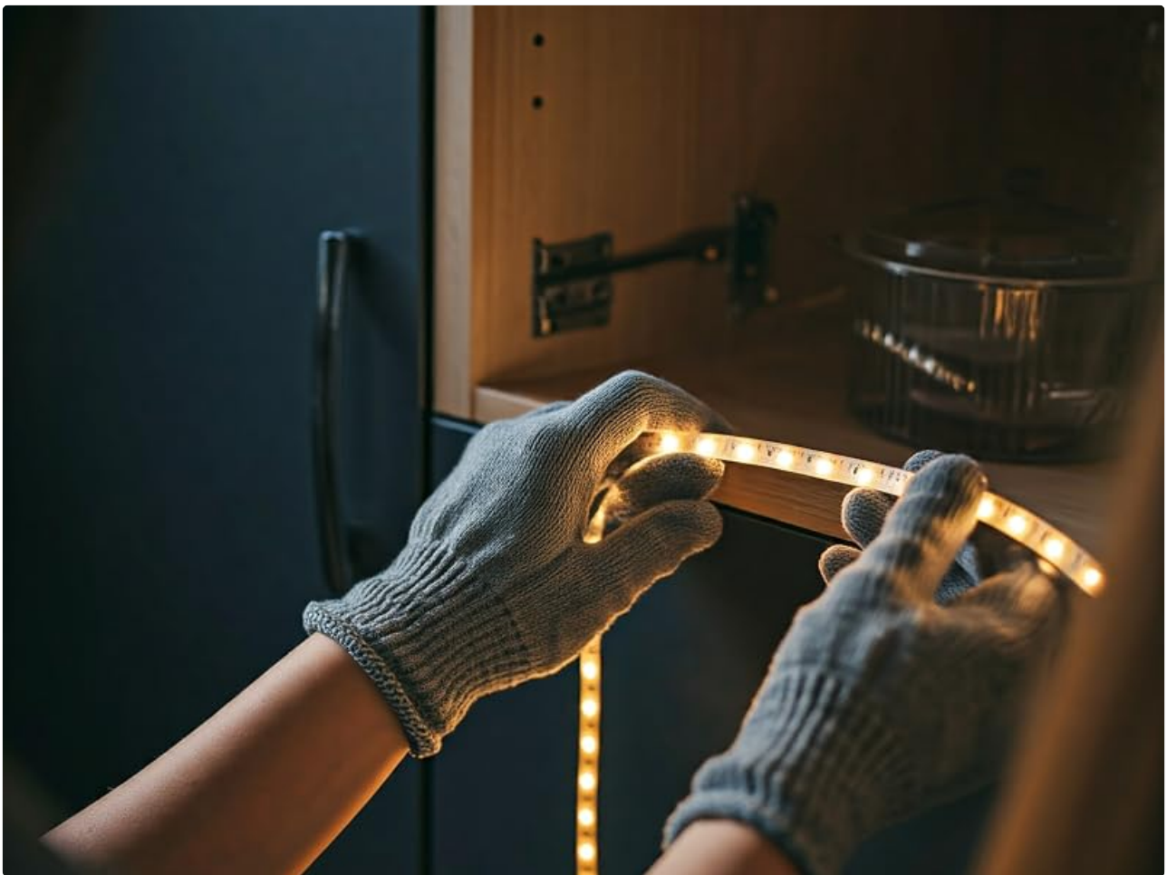
Image: An example of StripFlexLED installation, showing the lights applied under kitchen cabinets and shelves for accent lighting.
