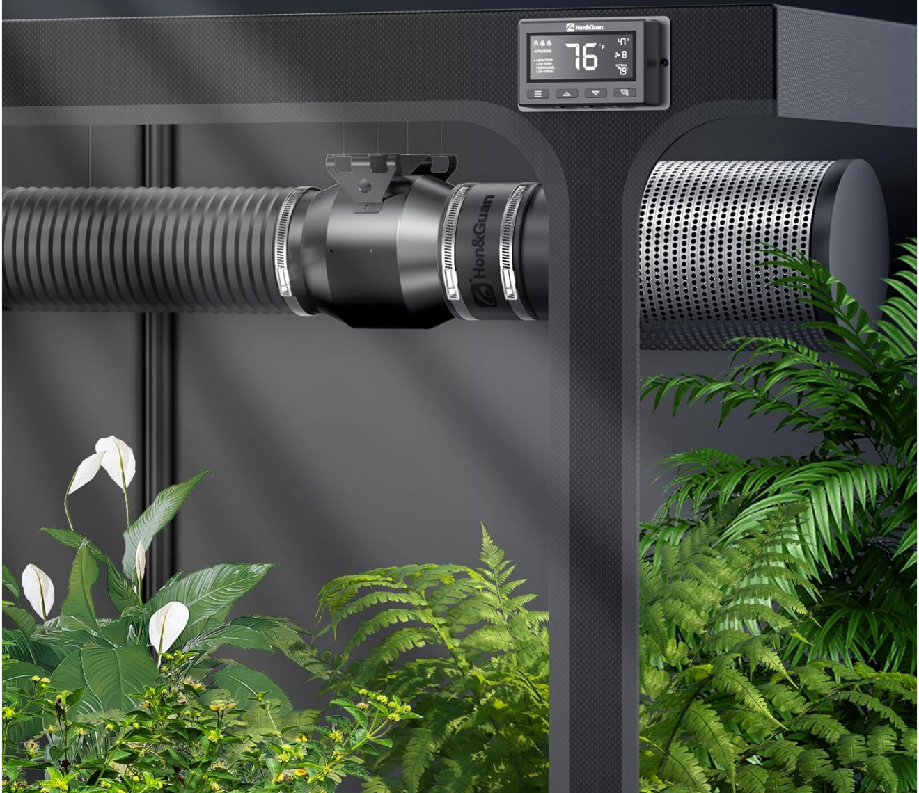
Image 3.1: Example installation of the ventilation system within a grow tent, showing the inline fan and carbon filter connected via ducting.
